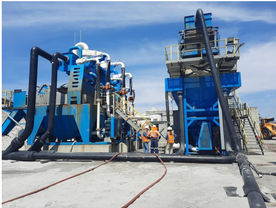
Plate 4 – Primary wash-screen process on right and dewatering units on left
